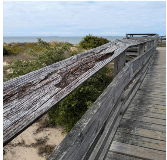
Figure 4: Deteriorated handrailing on boardwalk.
